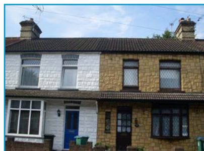
Inappropriate and ugly fake cladding
