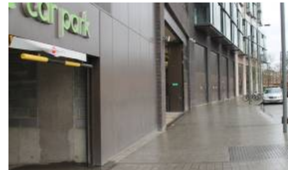
Car Parking provision can lead to dead and inactive frontages
