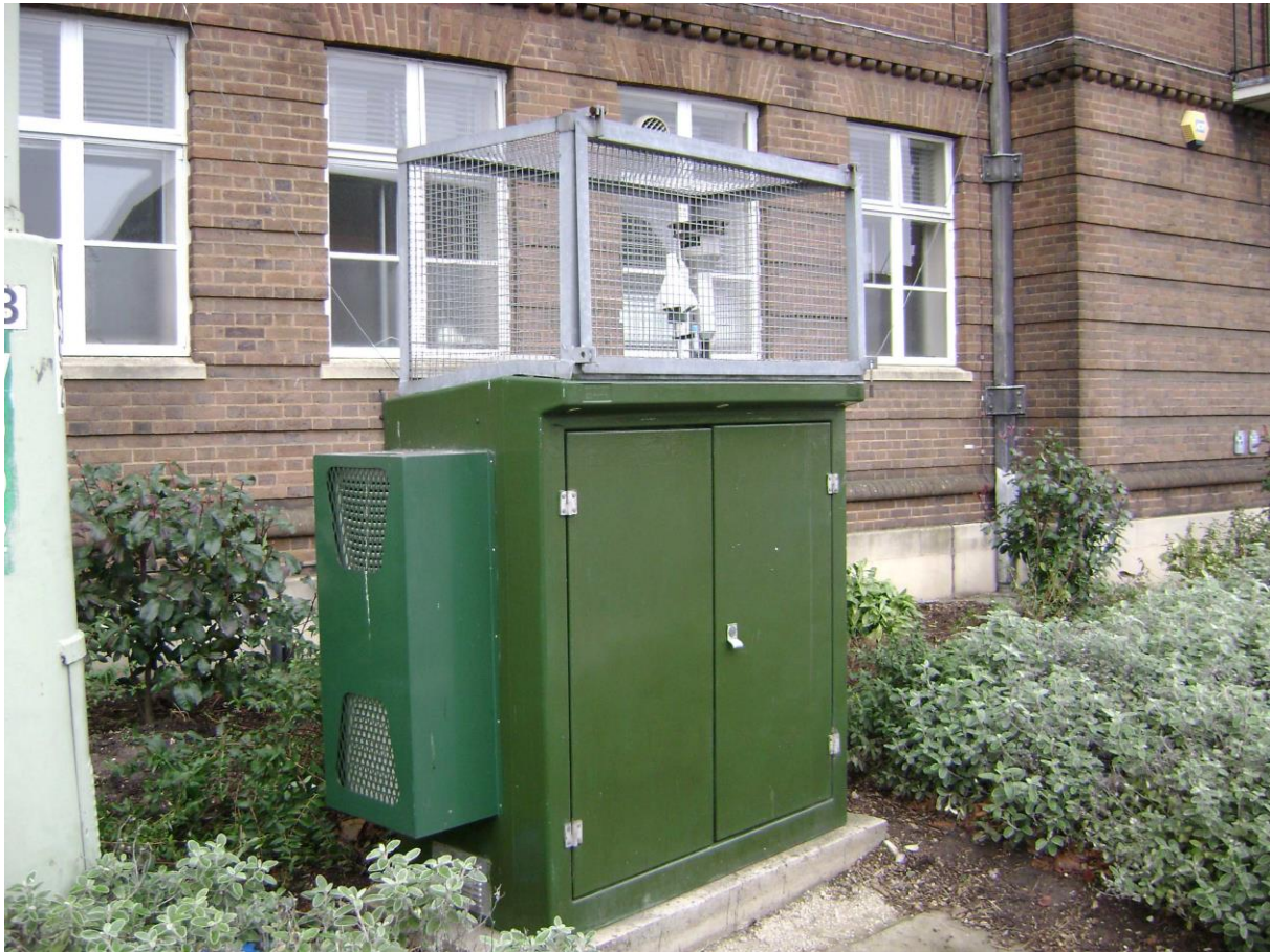
Figure 4: Photograph showing the automatic monitoring at Watford Town Hall.
